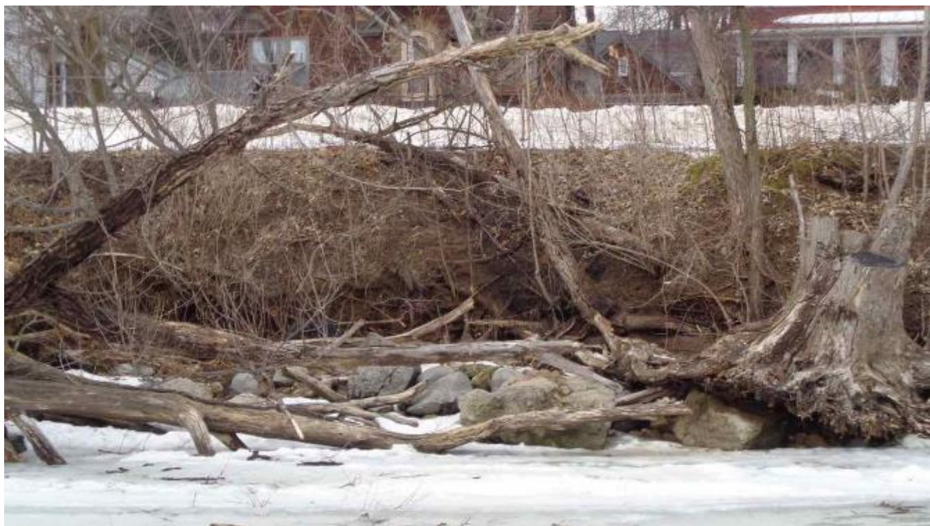
6. Example of slope collapse after trees were undercut. East of Hudson Beach.
